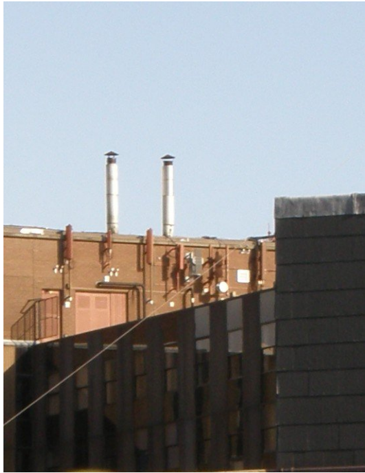
Transmitter Site Photo
