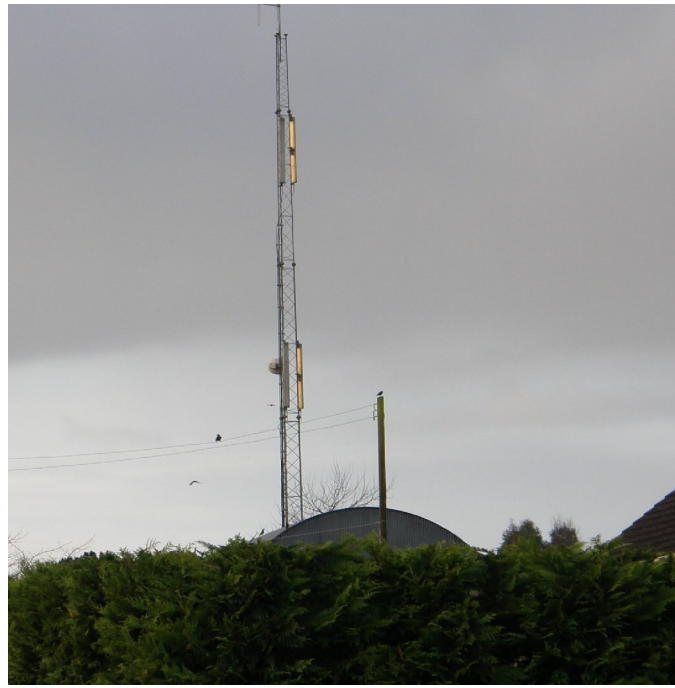
Transmitter Site Photo
