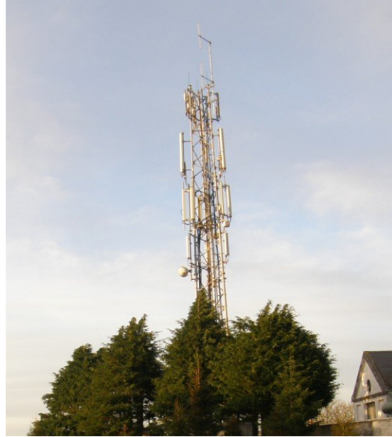
Transmitter Site Photo
