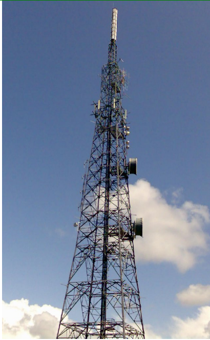
Transmitter Site Photo
