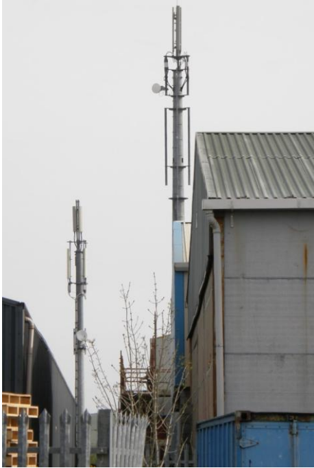
Transmitter Site Photo
