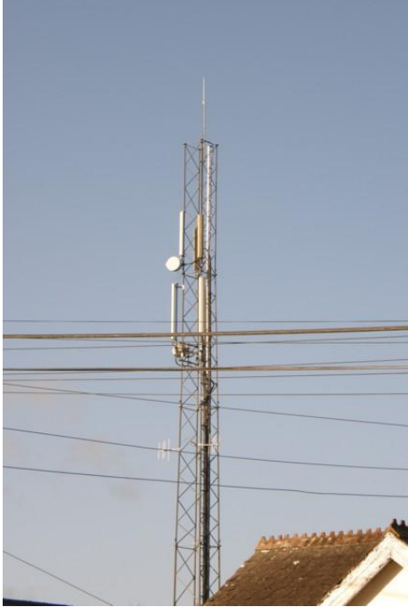
Transmitter Site Photo
