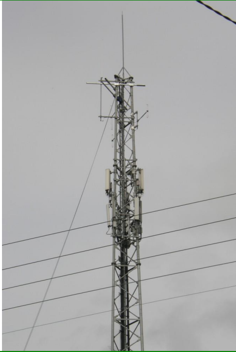
Transmitter Site Photo
