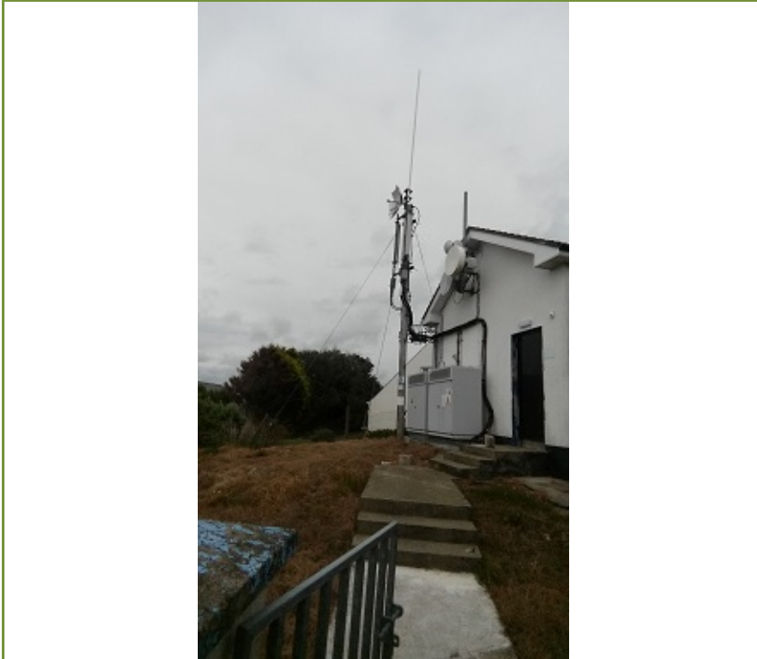
Transmitter Site Photo
