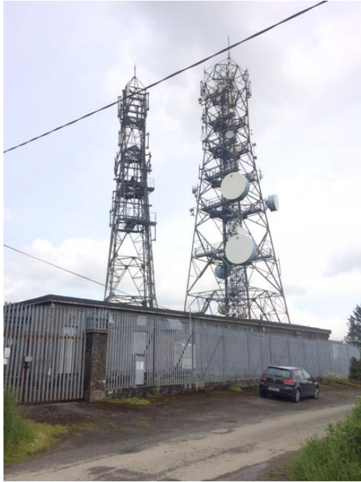
Designated Transmitter Site Photo
