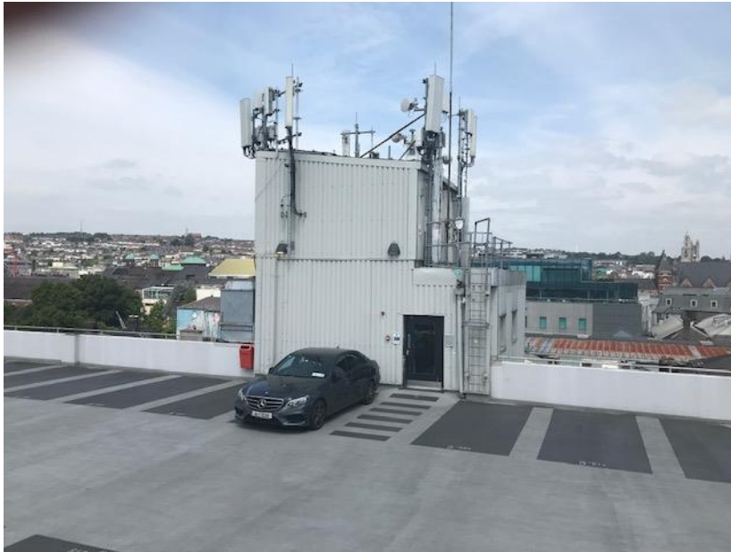
Designated Transmitter Site Photo
