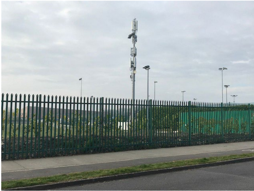
Designated Transmitter Site Photo
