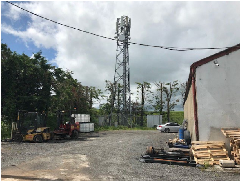
Designated Transmitter Site Photo
