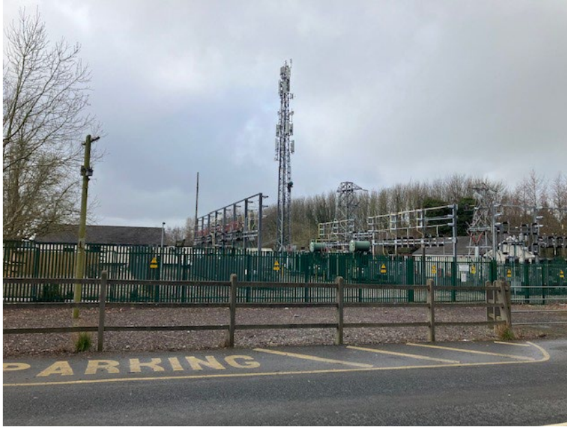
Designated Transmitter Site Photo
