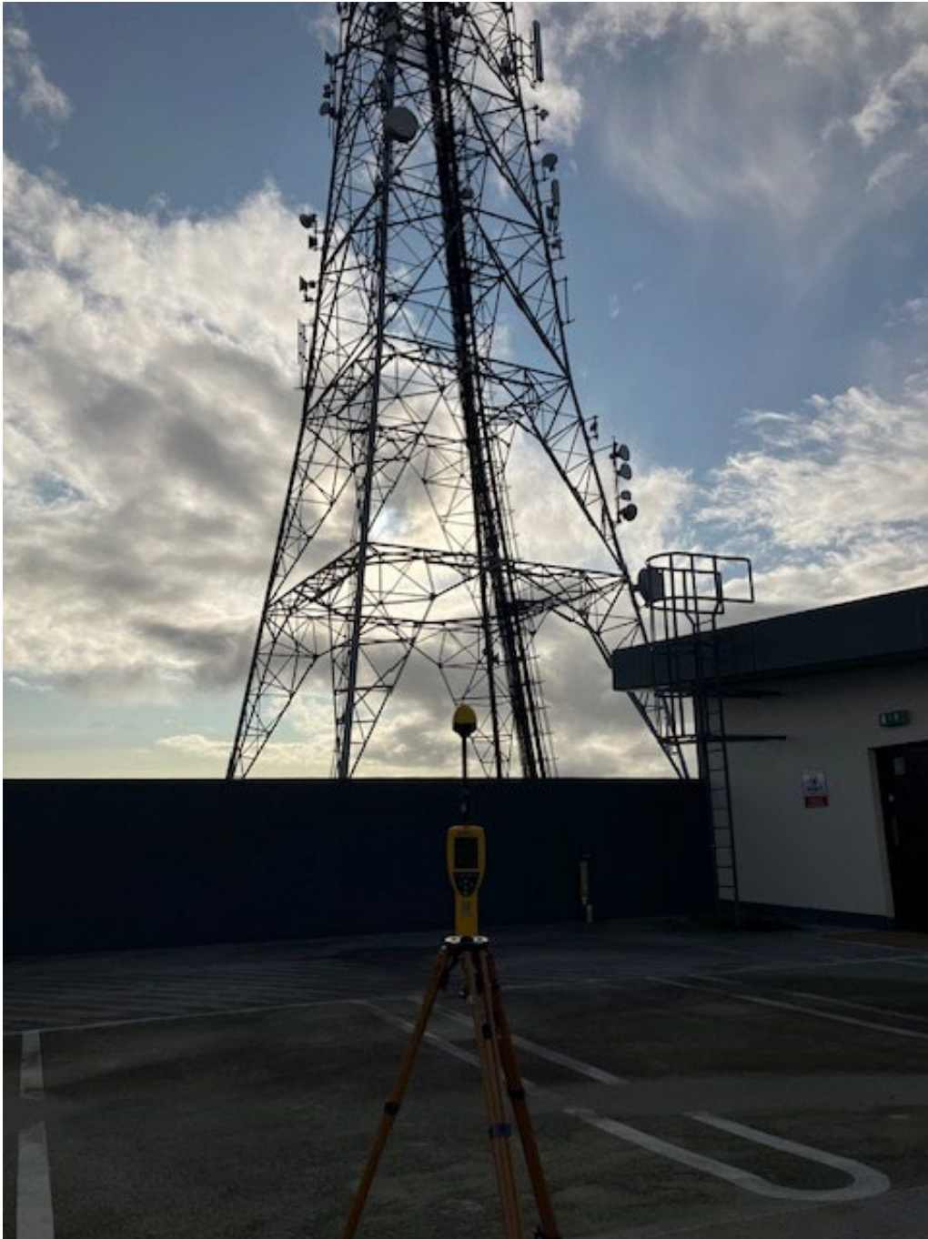
Photo 1. Broadband Measurement location looking towards antennas
