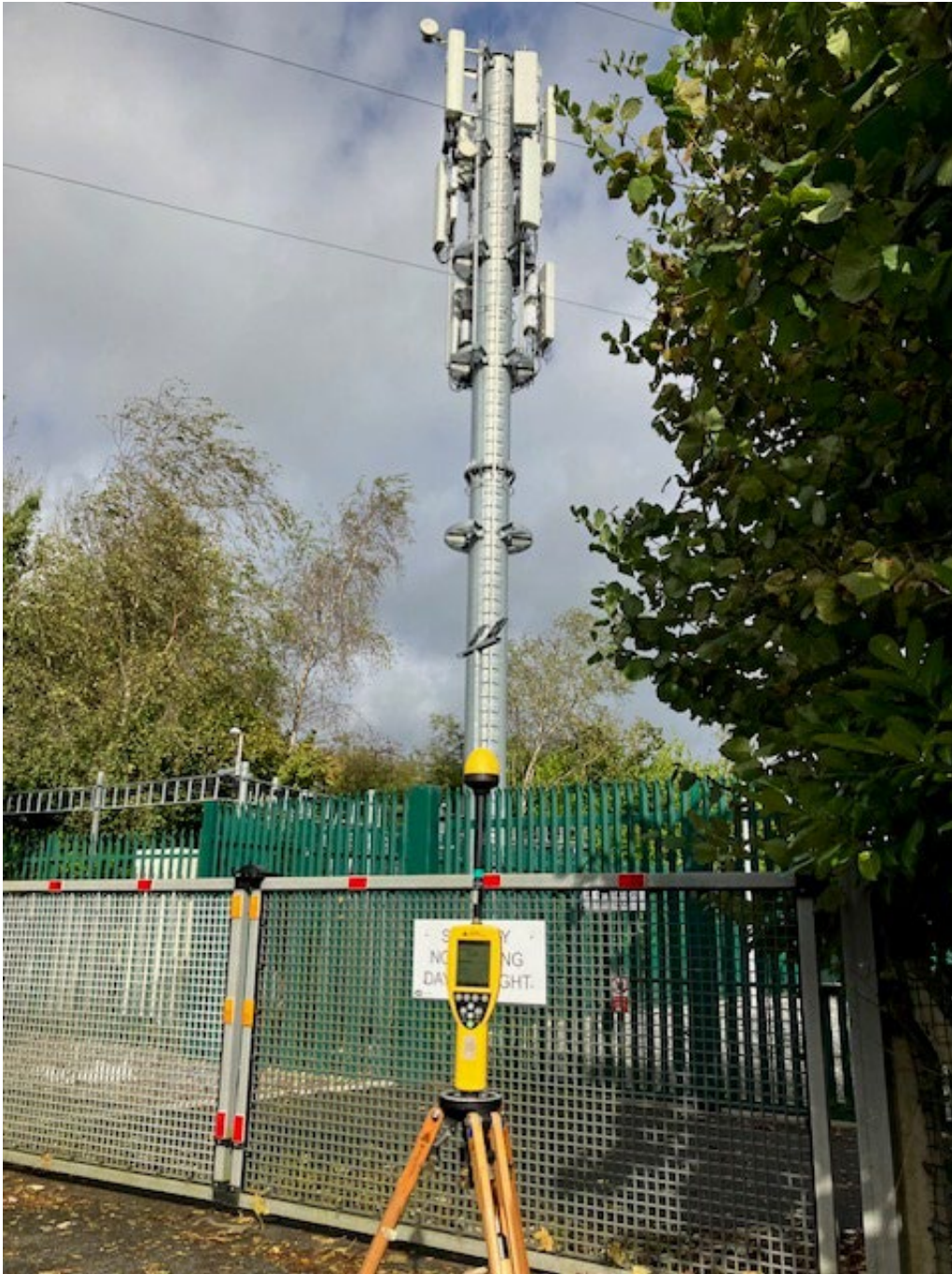
Photo 1. Broadband Measurement location looking towards antennas
